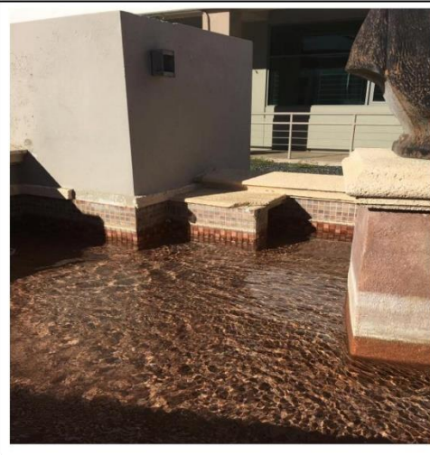
G-31 Plaza next to Coliseo; Damaged stone wall areas
