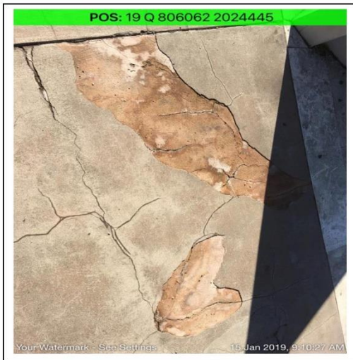
G-31 Plaza next to Coliseo; Damaged concrete walk area finish
