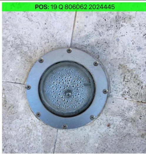
G-31 Plaza next to Coliseo; Typical non-working concrete floor light
