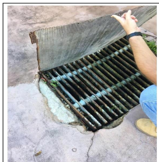
G-31 Plaza next to Coliseo; Damaged grate
