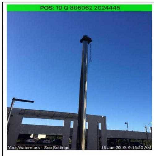
G-31 Plaza next to Coliseo; Pole with missing light; another pole with light is to left
