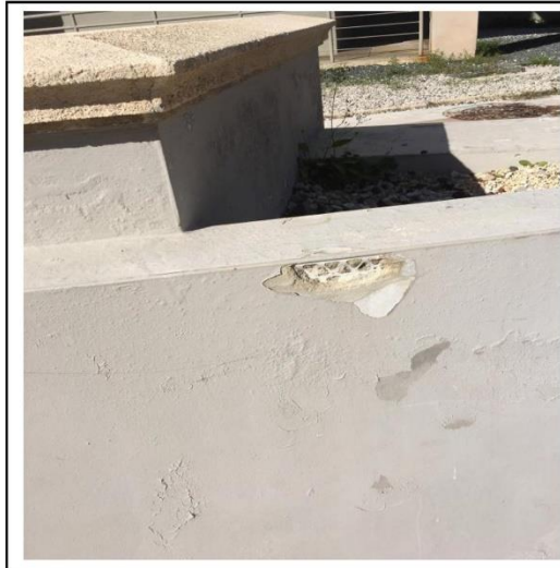
G-31 Plaza next to Coliseo; Typical damaged concrete wall plaster area
