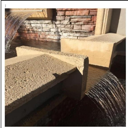
G-31 Plaza next to Coliseo; Damaged stone wall areas
