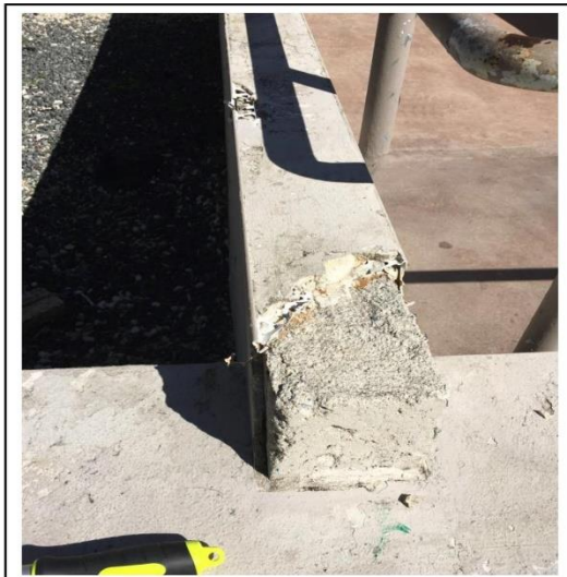
G-31 Plaza next to Coliseo; Concrete plaster damage
