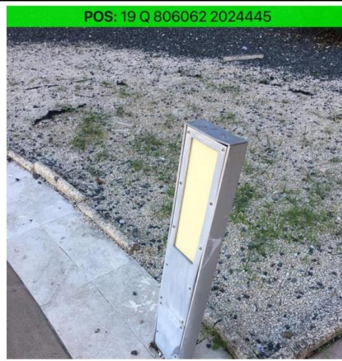
G-31 Plaza next to Coliseo; typical non-working walkway light
